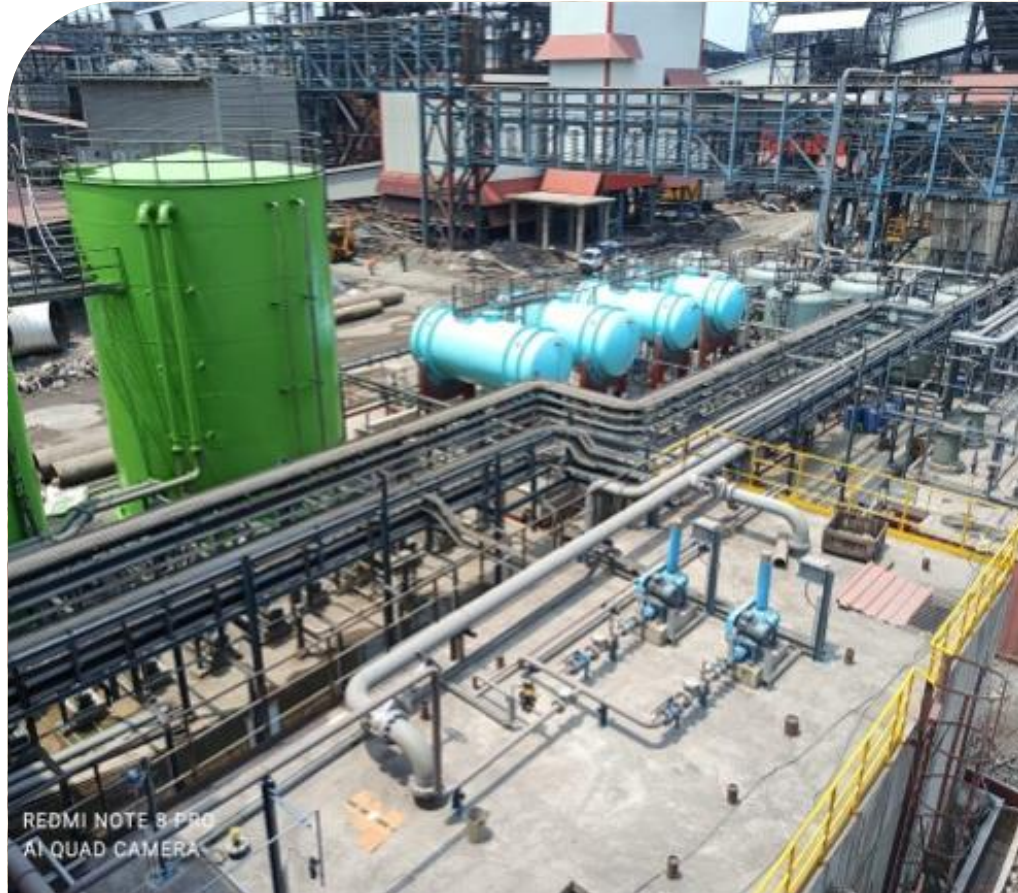
Pre-treatment Demineralisation plant for a steel major
