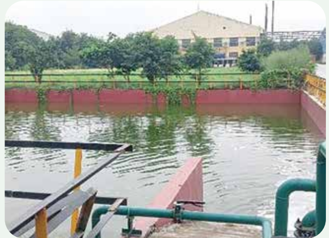
Rainwater Collection inside Bawal Plant Premises
