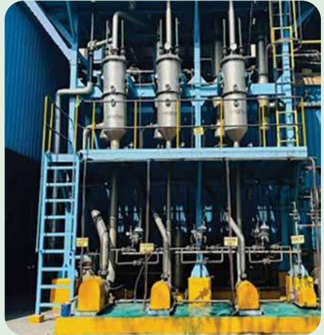
ZLD at Sayakha Plant
