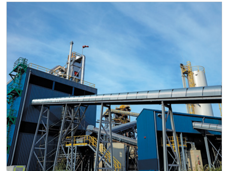
Hlsarna, a promising steelmaking technology with the potential of at least 20% reduction in CO 2 emissions and energy consumption
