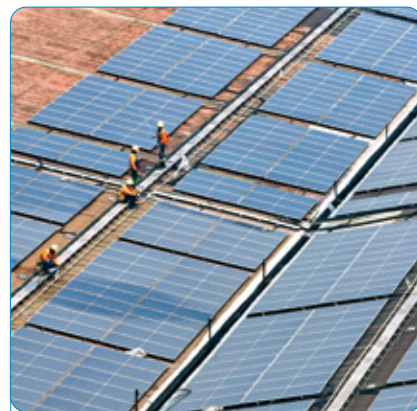
Rooftop solar installation at Hot Strip Mill, Jamshedpur plant
