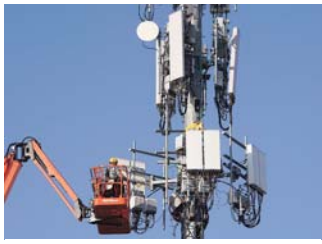
Companies have activated a comprehensive pandemic response plan with requisite risk mitigation protocols for keeping networks working as telecom is an essential service
