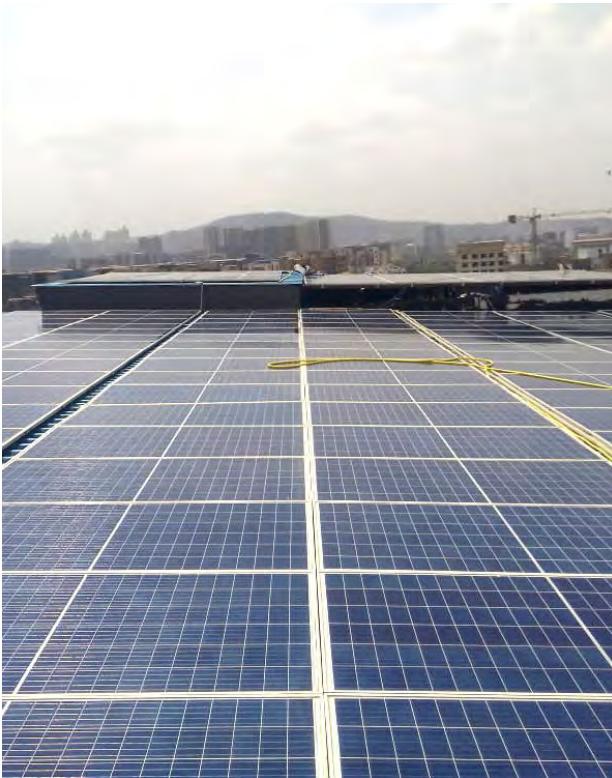
Vakrangee Corporate Office - Solar Panel
