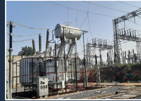
2 X 220 kV AIS bays at PGCIL Latehar, Jharkhand
