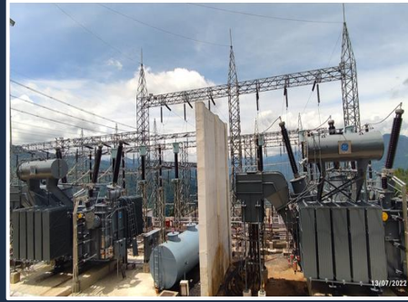
2nd 40 MVA, 220/ 33kV Transformer along with 33kV GIS for BPC at Dagapela, Bhutan
