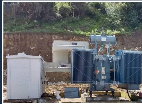
4 X 5 MVA, 33/ 0.415 kV Transformer Commissioned at BPC Damji, Bhutan
