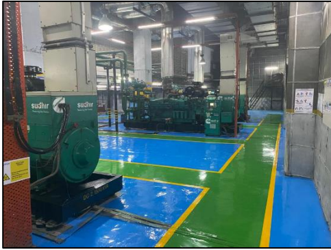
View of Block 9 & 10 DG Room
