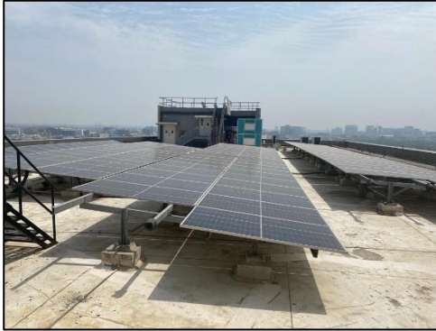
View of Rooftop Solar Panel
