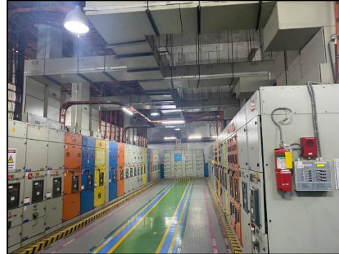
View of LT Room
