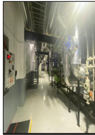
Internal View of Plant Room Tower 4, 5 & 6
