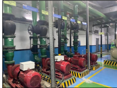
View of WTP & Fire Pump Room
