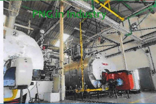
Natural Gas Skid
