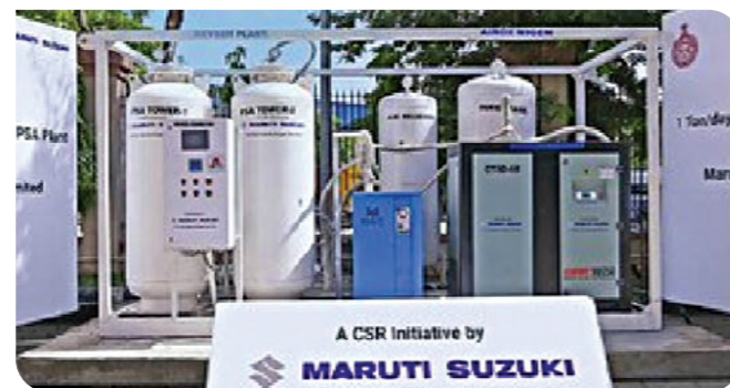
Oxygen PSA generation plant donated by the Company
