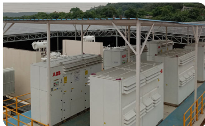
New solar plant at Manesar facility
