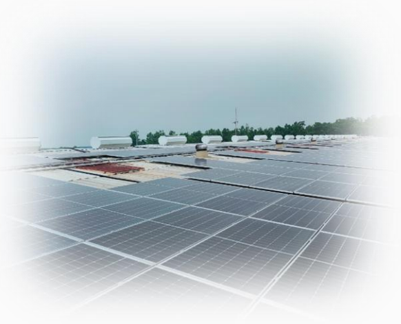
Roof-top solar at our Conductor plant in Orissa
