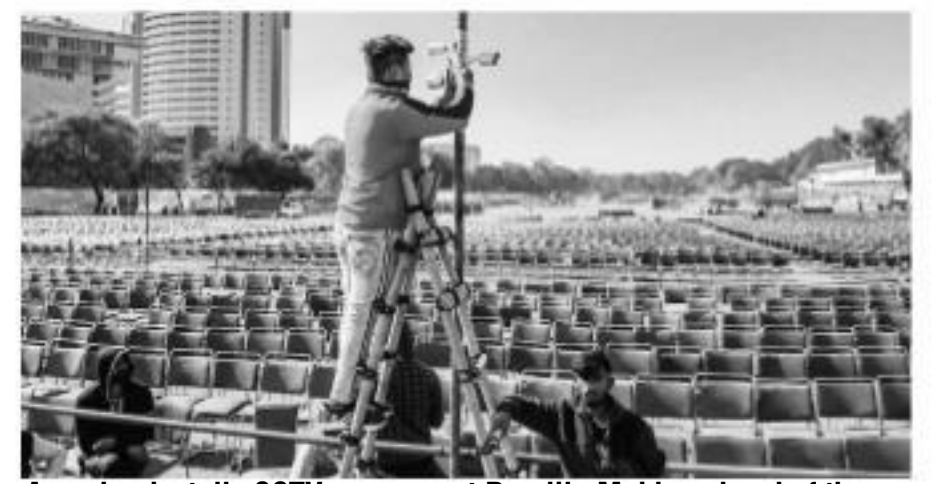
A worker installs CCTV cameras at Ramlila Maidan ahead of the oath-taking ceremony of AAP's government, in New Delhi on Friday
