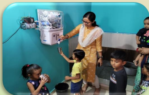
Successfully completed Aarogyam project; installed Domestic R.O/Water Purifier at Rahiyad Aanganwadi (Dahej) benefiting 45 Children
