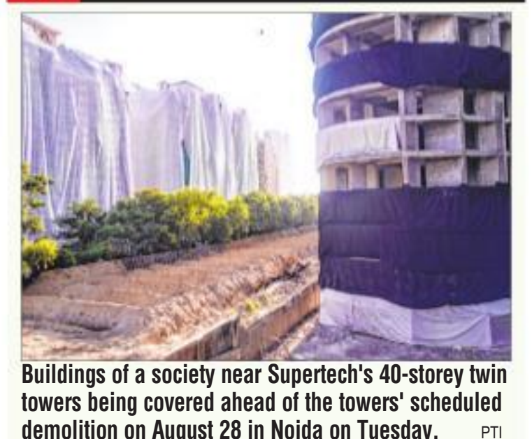
Buildings of a society near Supertech's 40-storey twin towers being covered ahead of the towers' scheduled demolition on August 28 in Noida on Tuesday. PTI
