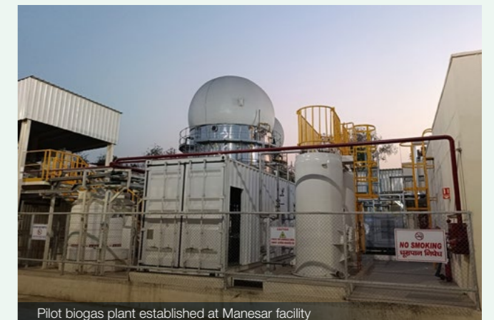
Pilot biogas plant established at Manesar facility
