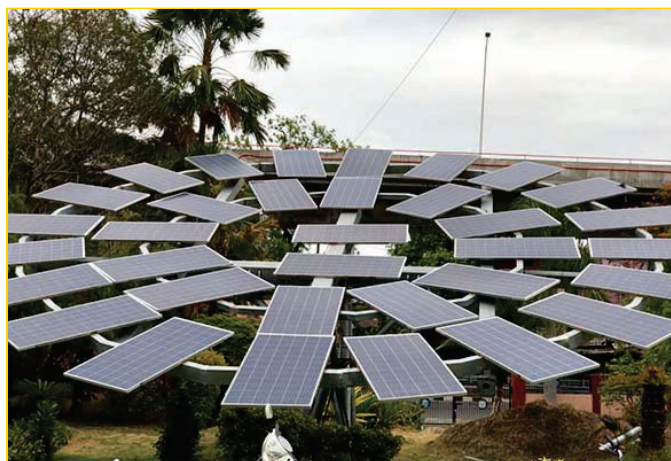
Solar tree installed at MOIL's Corporate Office
