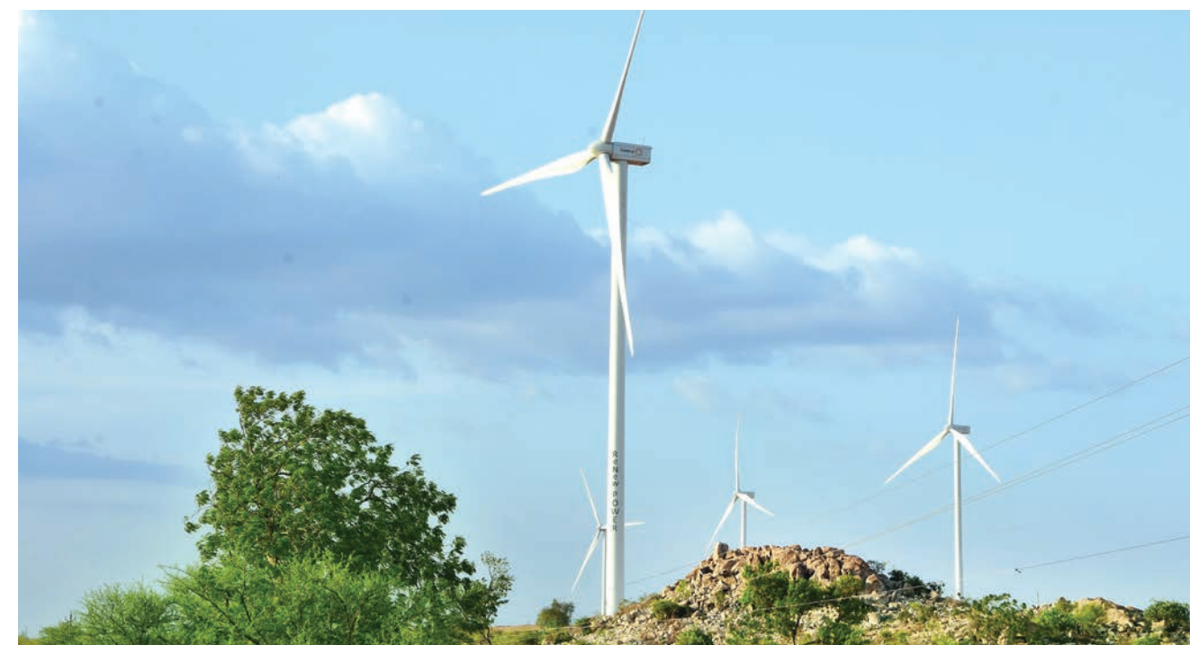
60 MW wind project of Renew Group in Karnataka, which was financed by REC
