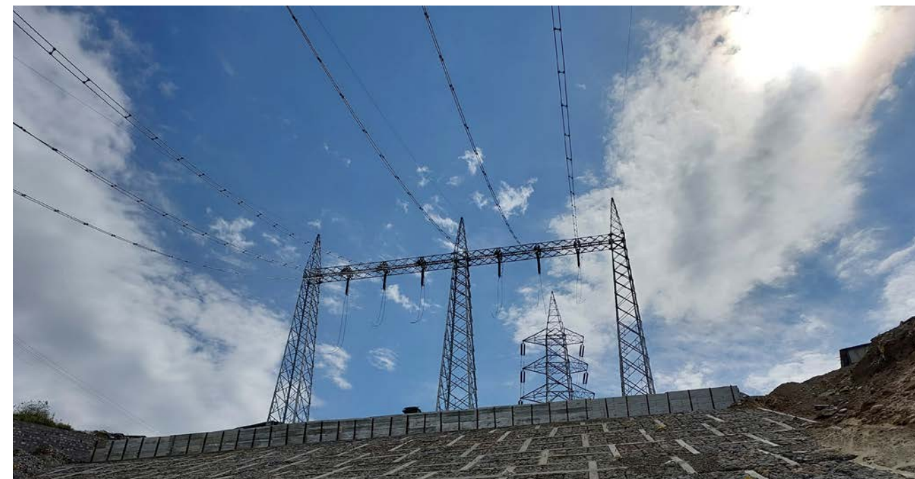
Switchyard at 2x60 MW Vyasi hydro electric project of Uttarakhand Jal Vidyut Nigam Limited, financed by REC
