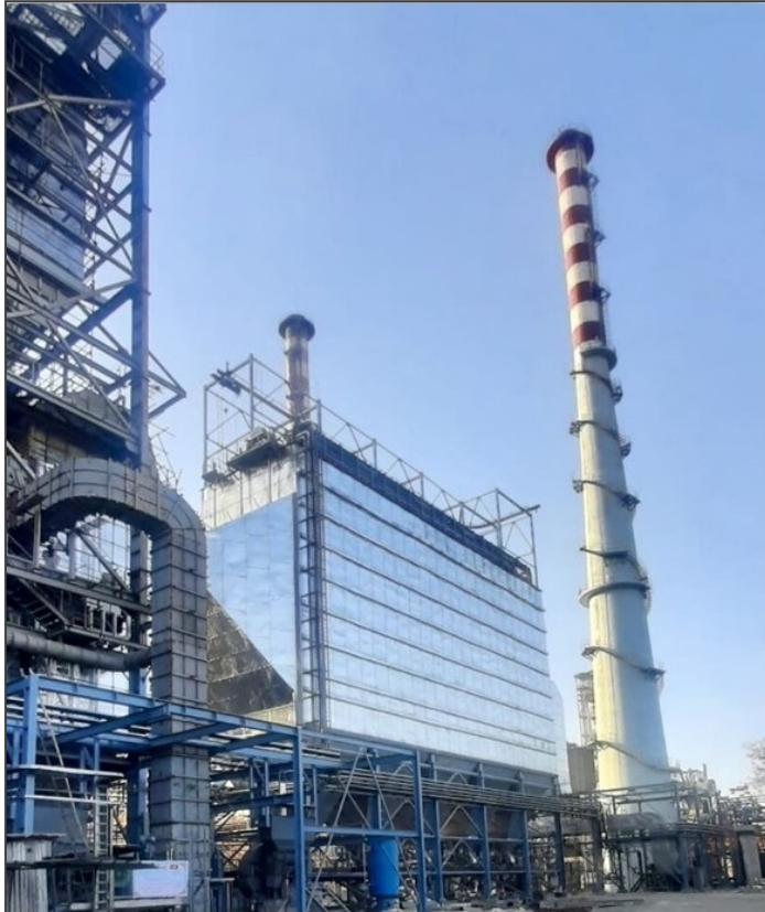
CFBC Boiler ESP for a leading cement company
