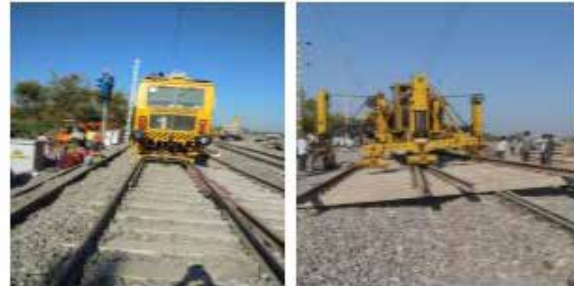
Connection of DFCCIL to NWR track at Karjoda station of Ajmer division – commissioned on 03.12.2020
