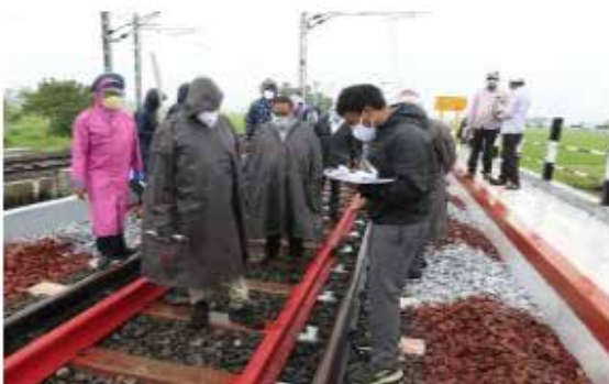
Commissioning of record 69 km (in one go) doubling work of Uppaluru – Moturu section and Gudivada- Machillipatnam section on 13.10.2020
