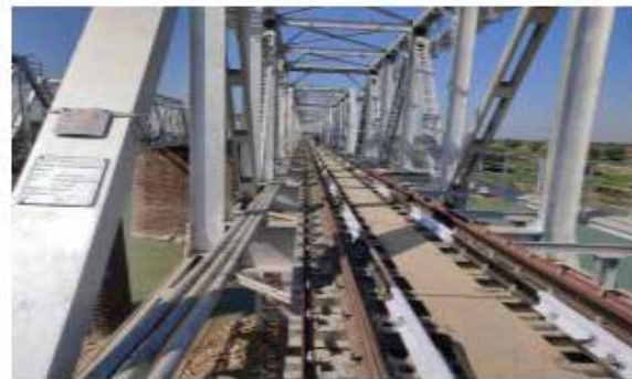
Commissioning of doubling work of Guna - Pilighata section over Bhopal Division on 29.12.2020
