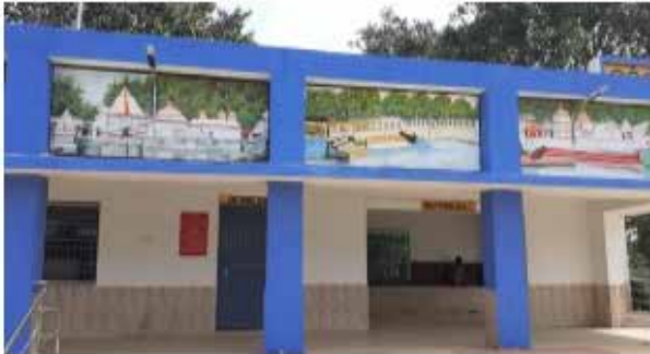
Commissioning of doubling work of 25 kms Lakhna - Hrishankar Road - Turekela Road section on 09.11.2020
