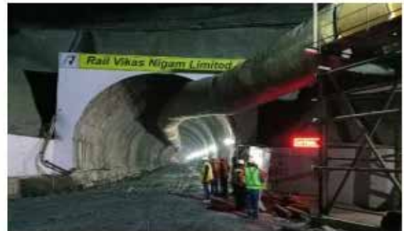
Completion of three adit tunnels of Rishikesh - Karnaprayag new railway line project
