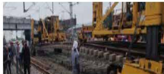
Commissioning of remodeled Mandideep Yard of Bhopal division of WC Railway on 14.07.2020
