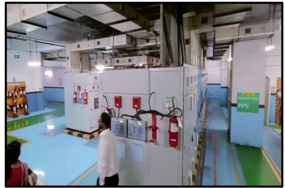
View of Electrical room
