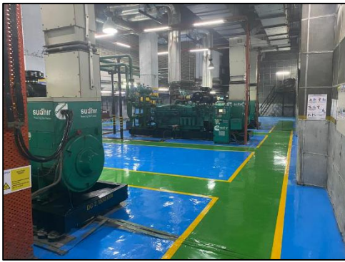
View of Block 9 & 10 DG Room
