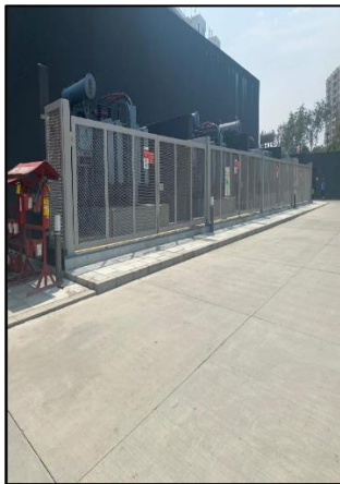
View of Power Back-Up
