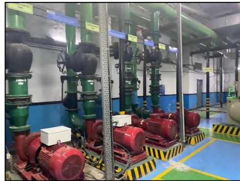
View of WTP & Fire Pump Room
