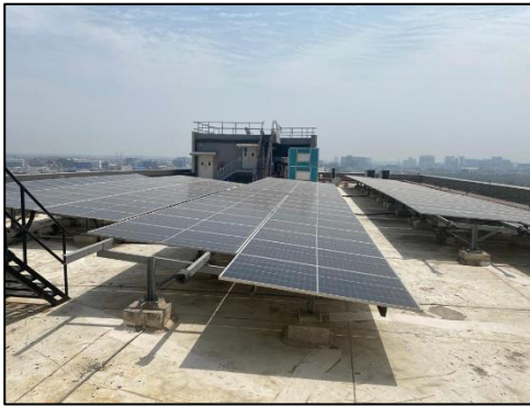
View of Rooftop Solar Panel
