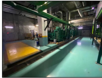
View of DG Room
