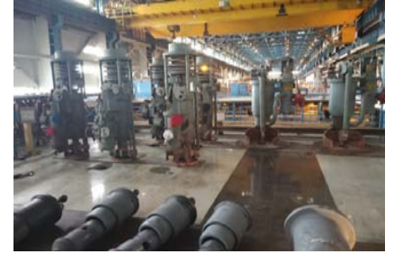
Control & Stop Valves Overhauling Sipat 660 MW
