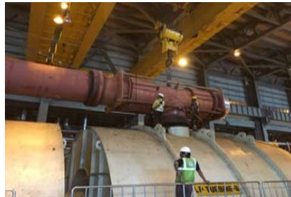
Turbine AOH, 600 MW, Udipi
