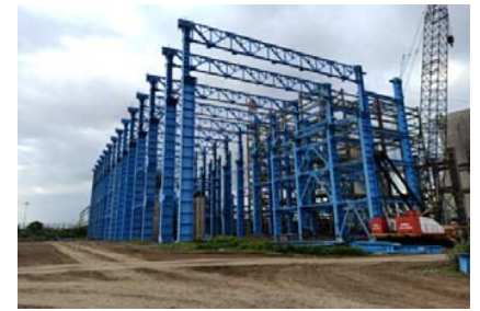
1X660 MW Bhusawal TPS at Maharastra-MAHAGENCO
