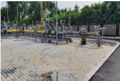
Station Piping at Ennore, IOCL
