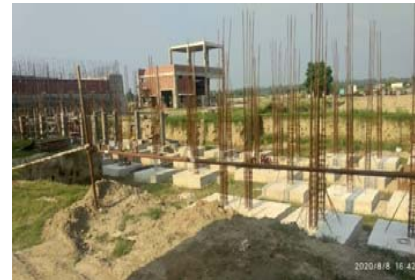
28 MLD STP at Karnal, TPL
