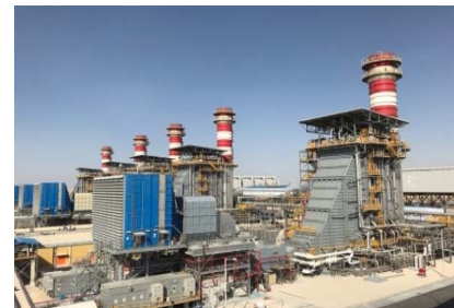
1,519 MW Fadhili CHPP, Doosan, KSA
