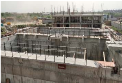
27.5 MLD STP, Networking at Palwal, MCPALWAL
