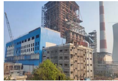
1x800 Mw TPSS, North Chennai, TNNGEDCO
