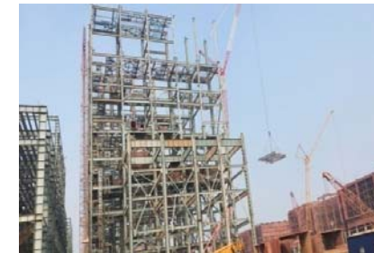
5x800 MW Yadadri TPP, TSGENCO
