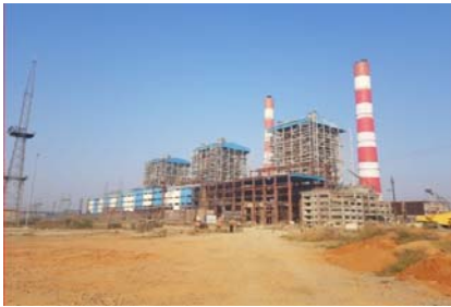
3x660 MW Nabinagar STPP, NPGCL
