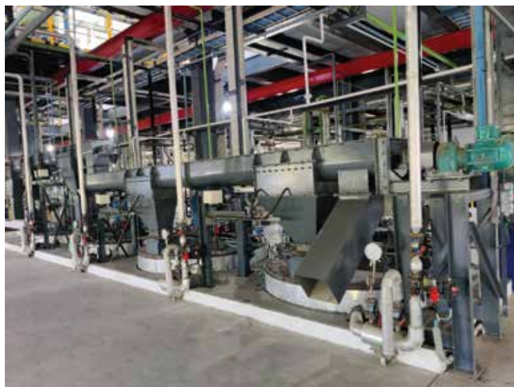
New sulphur black facility
