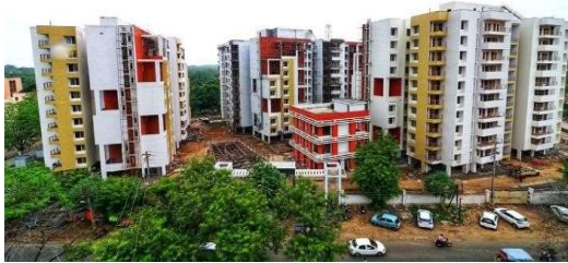
Construction of 222 Flats at Keelandev Tower, Bhopal for MP Housing & Infrastructure Development Board
