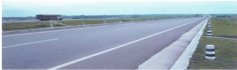
Maintenance of NH-19, (earlier NH-2) Barwa Adda – Panagarh Section (KM 398.75 –KM 512.00) in the state of Jharkhand & WestBengal
