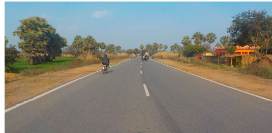
Upgradation of roads and bridges of Shivganj-Rafiganj-Goh-Uphara-Devkund-Baidrabad Road (SH-68, in the state of Bihar)
