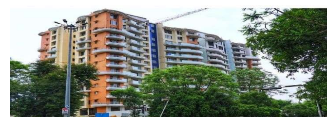
Construction of 96 flats at Tulsi Tower, Bhopal for MP Housing & Infrastructure Development Board
