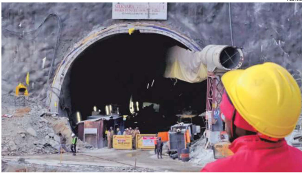
A worker on Wednesday overlooks the entrance of the tunnel where 41 men have been trapped for over 10 days
