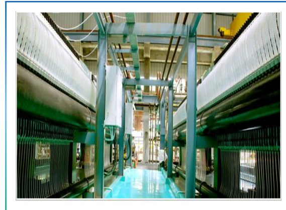
Caustic Soda manufacturing, Karaikal, Puducherry
