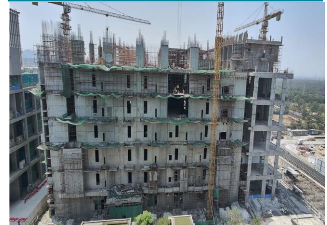
Mindspace Airoli West Building 8- Data center – 0.3 msf Estimated Completion : Q4FY25
