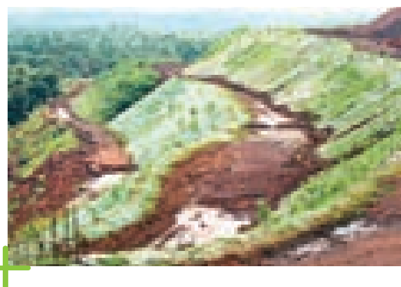
Below: Geotextile laid on dump slopes for dump stabilisation at Codli mine
