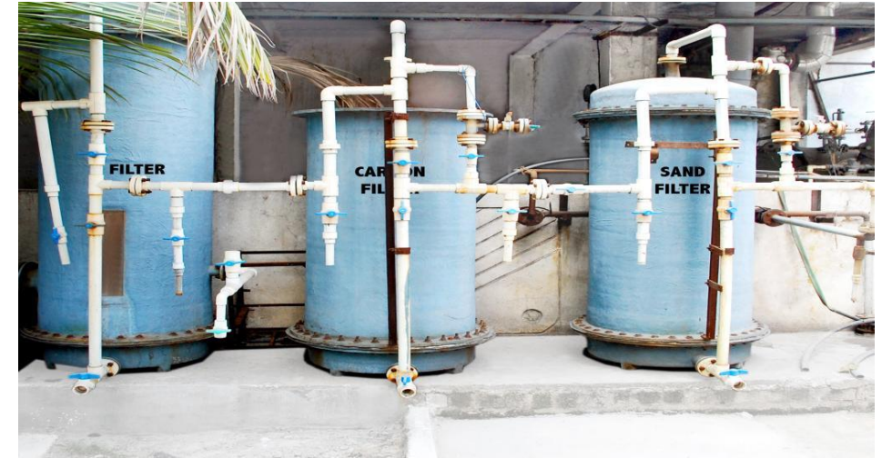
(Reverse Osmosis Plant) R.O. Plant
