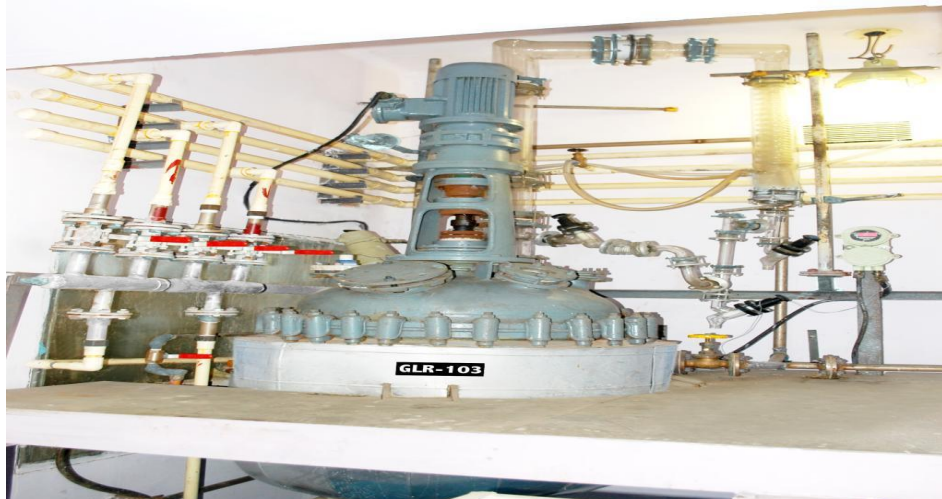
Glass Lined Reactor
