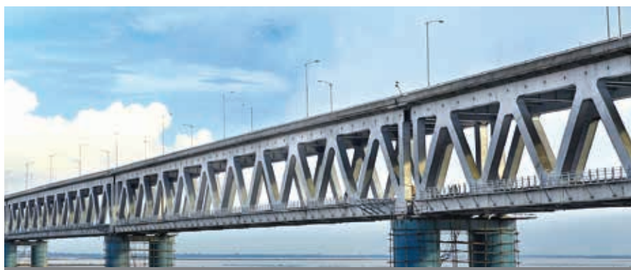
Bogibeel bridge over brahmaputra river in assam coated with AP-PPG Coatings, EPC contractor HCC
