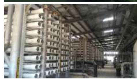
50 MLD BWRO (Desalination), for Reliance Industries, Dahej, India Turnkey project executed in record 8 months 24 days
