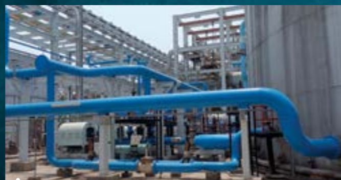
All pipelines, caustic vessel, filter vessel in refinery are coated with high performance surface tolerant epoxy PROTECTOMASTIC system with BERGERTHANE as topcoat.
