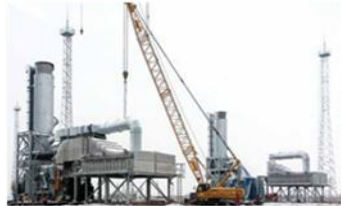
35 MW GT POWER PLANT, KAZAKSTHAN
