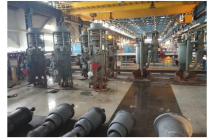
CONTROL & STOP VALVES OVERHAULING SIPAT 660MW
