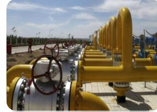
City Gas Distribution
