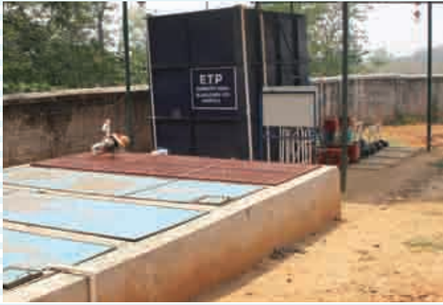
Effluent Treatment BIO-Plant at Rourkela
