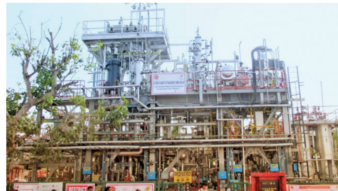
Hydrogen CNG plant at Rajghat, New Delhi
