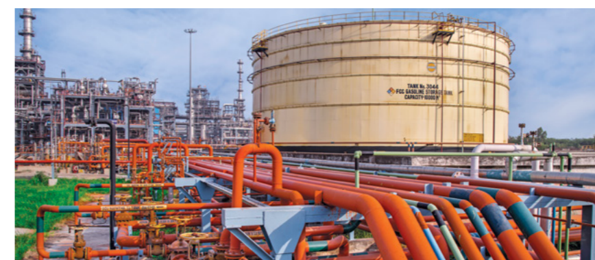
IndianOil owns and operates over 15000 kms of pipelines to reach its energy supplies to the customer touch points
