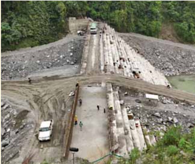
Coffer Dam & Intake Structure Work is in Progress at 900 MW Arun - 3 HEP, Nepal
