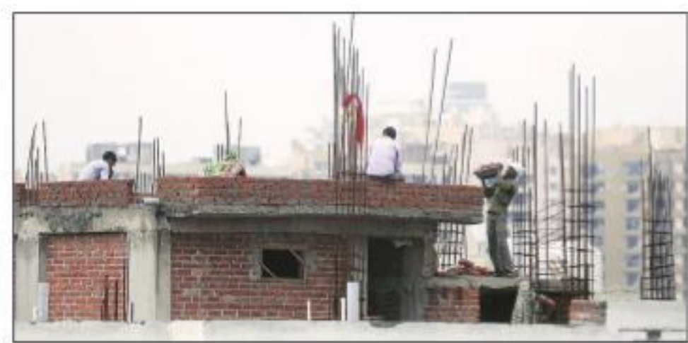
More than 1,400 buildings are under scanner. Abhinav Saha
