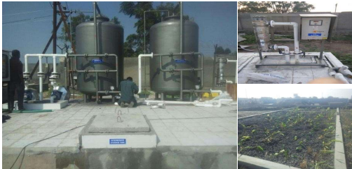
Sara Builders & Developers Pvt. Ltd. - 500 CMD STP
