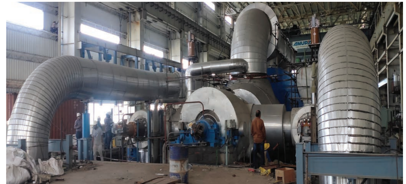
REC financed 800 MW Dr. Narla Tata Rao Thermal Power Station Stage-V Project at Vijayawada
