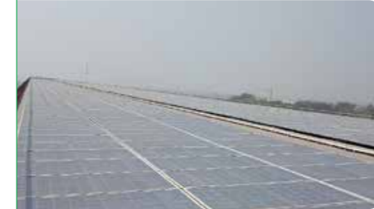
Commissioning of WHRS 8.80 MW and 1.25 MW solar power
