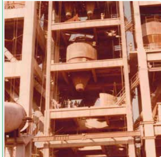
Installed a KIDS cooler, which is a clinker inlet distribution system
