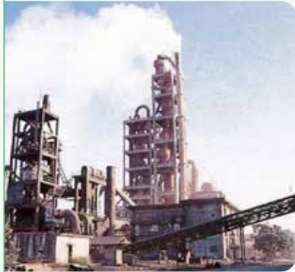
Installation of separate line calciner with five-stage pre-heater and jaw crusher
