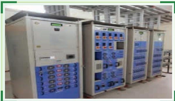
IPS Room, Moradabad S&T Project
