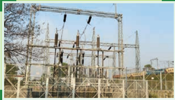
132 KV Cable termination at Lalkuan TSS end, RE PKG-5
