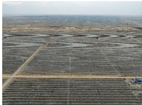
Bi-facial solar modules installed at Khavda
