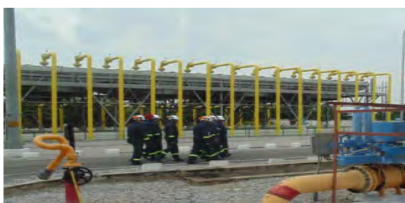
CS - 3 Gas After Cooler
