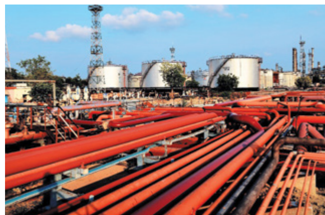
IndianOil is a pioneer in petroleum pipelines in the country and manages one of the world's largest energy pipeline networks
