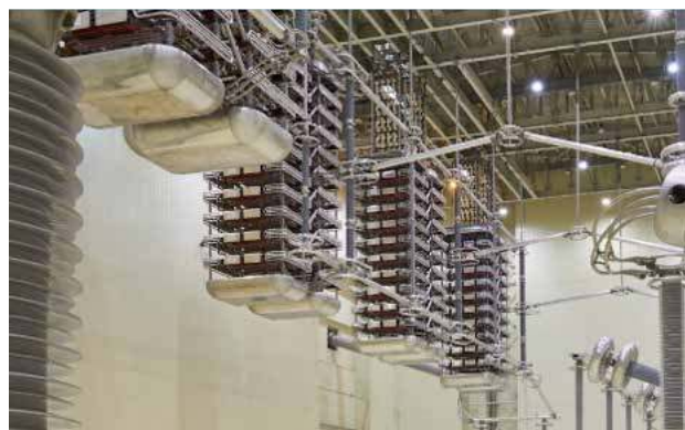
Commissioned Pole-4 of Champa Kurukshetra Phase-2 project for PGCIL. With commissioning of the fourth pole, the capacity of Champa-Kurukshetra transmission link has increased to 6000 MW
