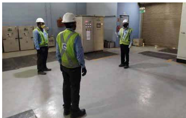
Services team of GE T&D Grid Solutions worked round the clock to ensure uninterrupted delivery of power supply at Delhi & Chennai airport
