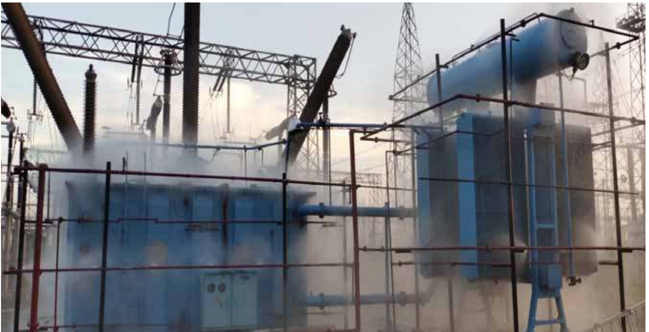
400 kV 125 MVAR bus reactor for NTPC at Kahalgaon
