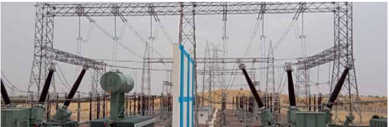
Three 132 kV Air Insulated Switchyard (AIS) bays commissioned for Sterlite in North Eastern Region Substation package at Surajmani Nagar
