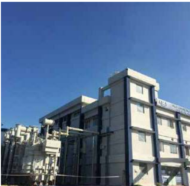
220 kV Gas Insulated Substation (GIS) bays and 160 MVA Transformer commissioned for Kerala State Electricity Board (KSEB) at Kaloor
