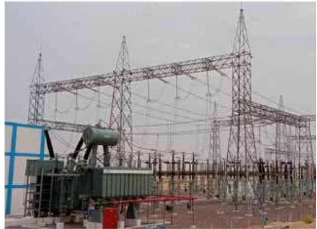
Energized 400kV GSS, RSS with 150MVA Trafo & 12x12.5 MW ICRs for Azure Power at Bikaner
