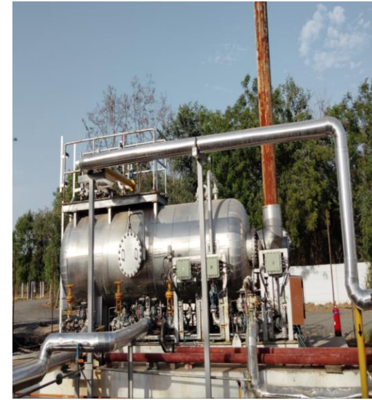
Karjisan Surface Facility Heater Treater area
