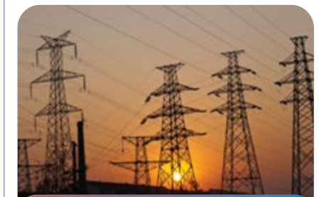
Transmission system in Rajgarh II (BOOT)
