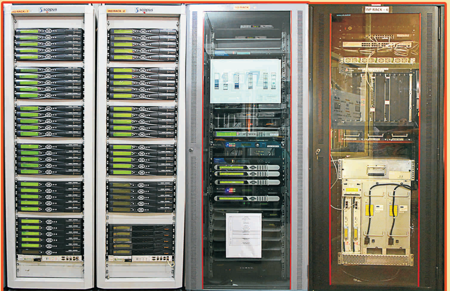
State of the Art Network Operating Centre at Bhubaneswar
