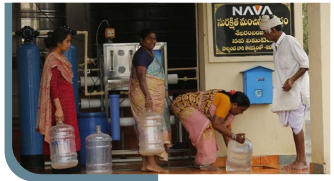
Safe Drinking Water Plant
