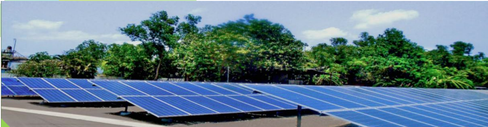
Solar Panels at Roha
