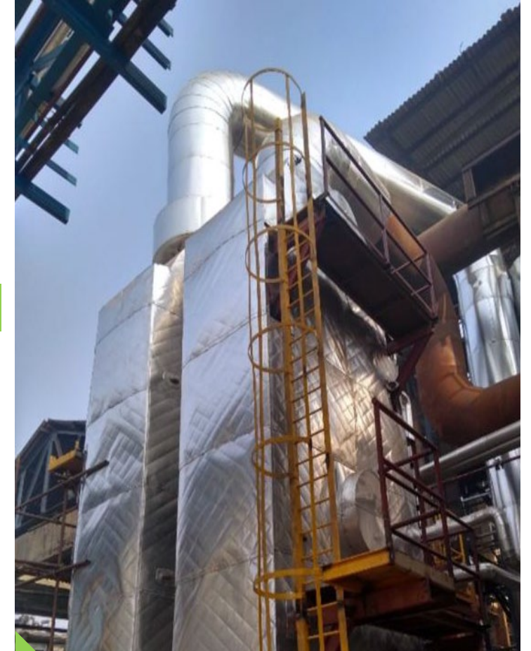
Waste heat recovery system
