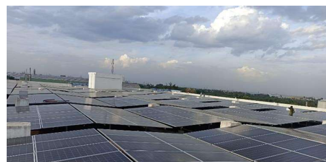
Rooftop Solar installed and commissioned at 9 manufacturing plants
